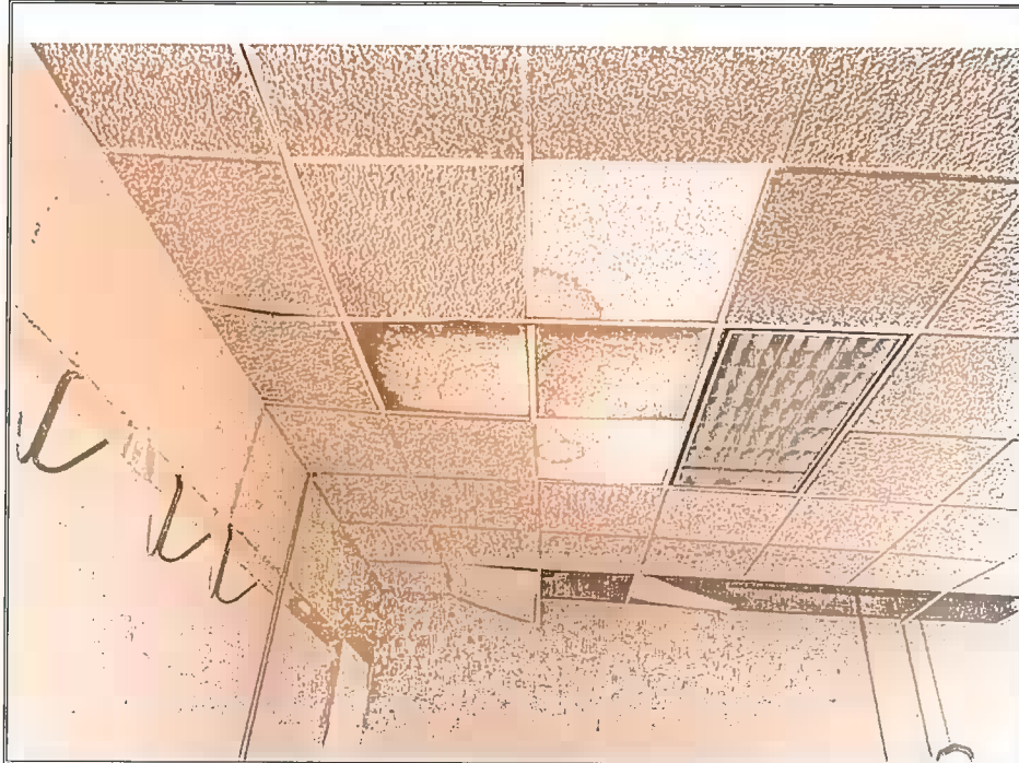
WATER STAINS ON CEILING TILES
