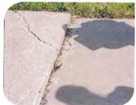
This sidewalk change in level is greater than 1/4 inch, not beveled or flush, which can be hazardous for those walking or rolling across it.
