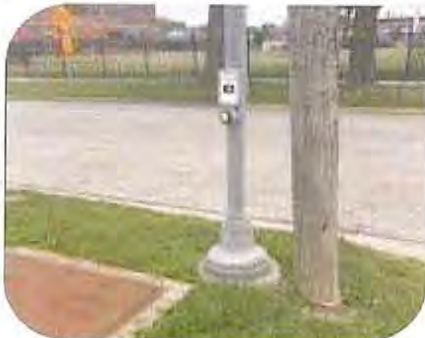
This pedestrian crossing button can't be reached from the sidewalk. The button is too far away, facing the wrong direction, and obstructed by another pole.
