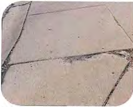
This sidewalk crossing has excessive cross-slope and deterioration, which can be challenging to walk or roll across.
