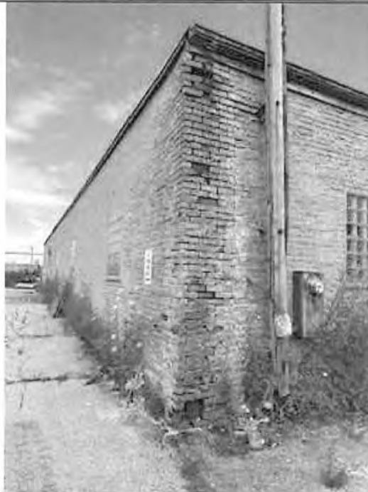
SOUTHEAST CORNER OF BUILDING IN NEED OF MASONRY REBUILD
