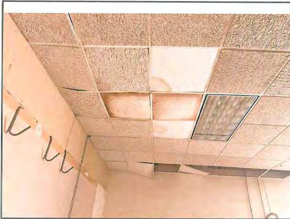
WATER STAINS ON CEILING TILES
