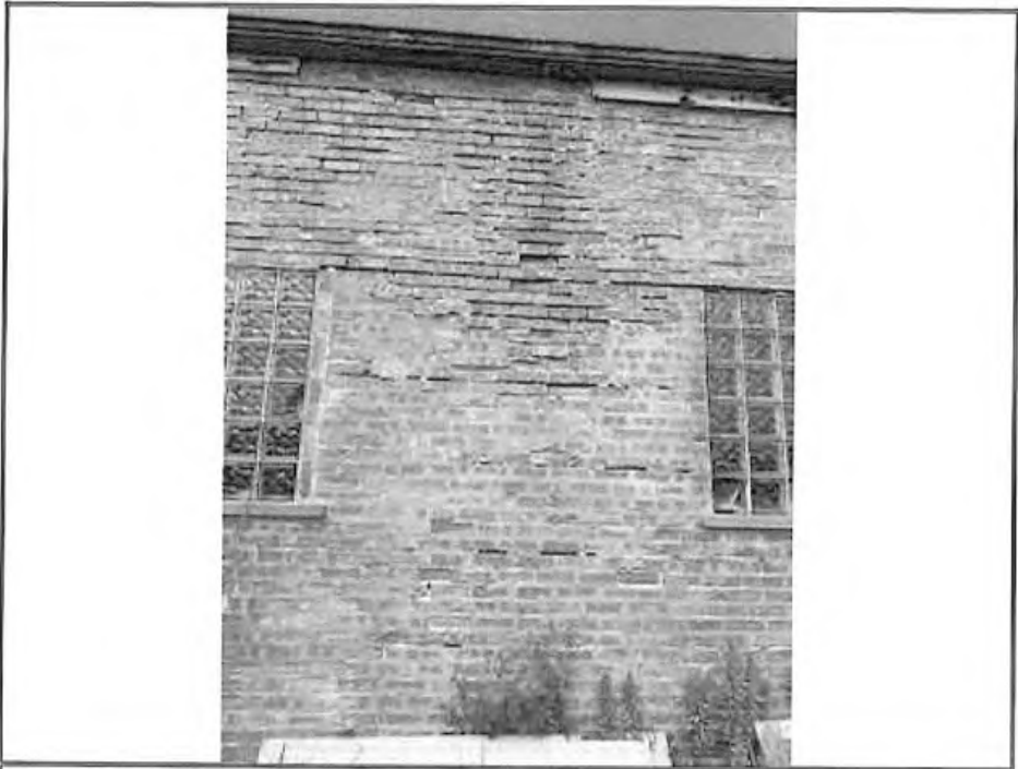
AREA IN NEED OF MASONRY WORK
