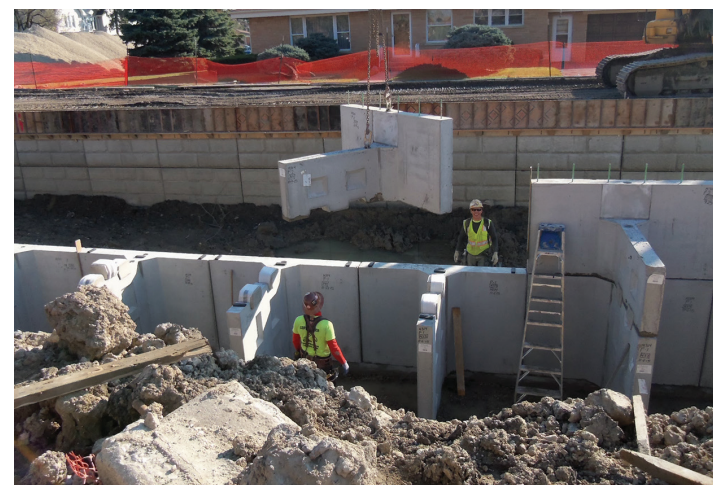
▲ Engineers and construction crews continue to make progress on the Silver Creek Channel Improvement project. Check our website at vofp.com for updates.
