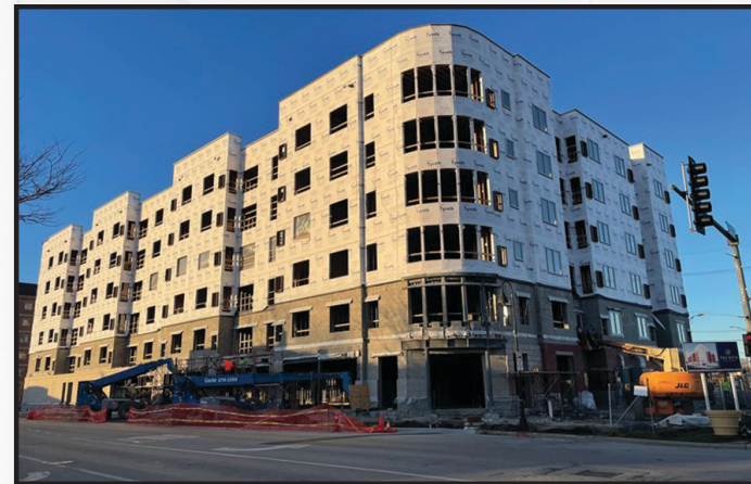
▲ Construction on Phase II of the Crossings development is continuing with the construction of a new 110 luxury unit market rate rental building at 9600 Franklin Avenue.
