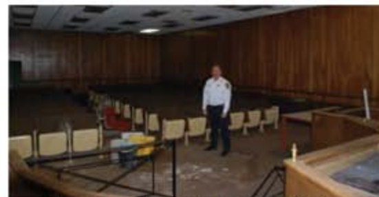
Franklin Park Police Chief Michael Witz scatters buckets throughout Police Station to capture water leaking from the roof.
