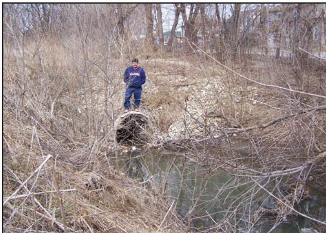
Joe Thomas inspects the Schiller Park restrictor on Crystal Creek
